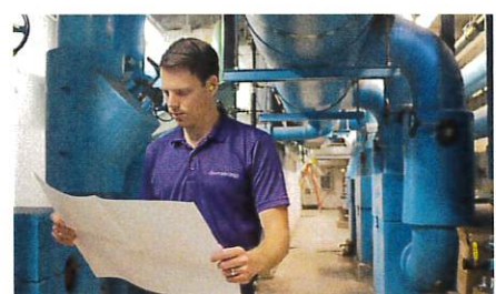
MECHANICAL, ELECTRICAL, PLUMBING
