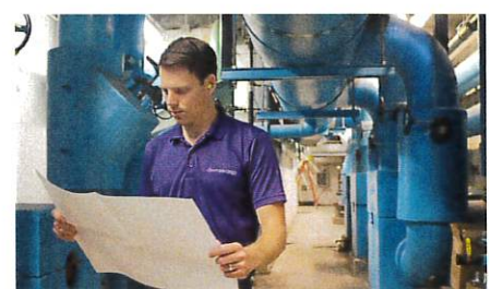
MECHANICAL, ELECTRICAL, PLUMBING
