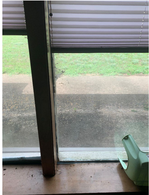
Above: Deteriorated window frame at 1157 Nichols Rd.
