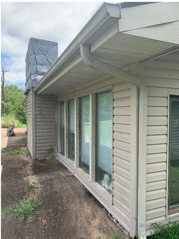
Above: Deteriorated window frame and chimney at 1157 Nichols Rd.
