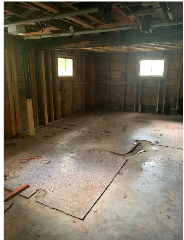
Above: Deteriorated walls at 1167 Nichols Rd.
