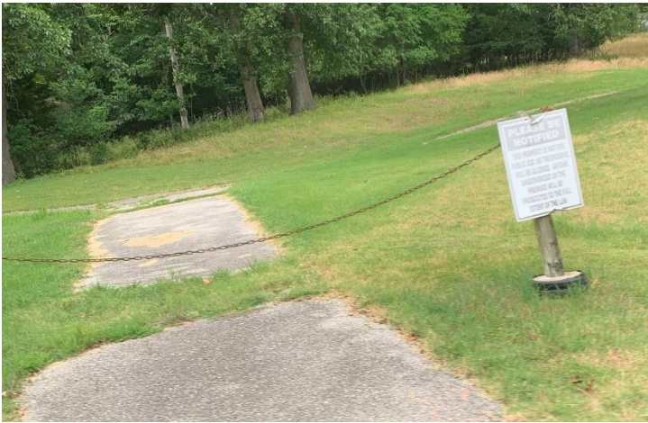
Above: Deteriorated golf cart path.
