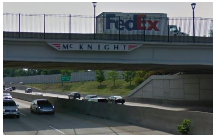
FIG 3.4.2: SIGNAGE ATTACHED UNDER BRIDGE OVERHANG
