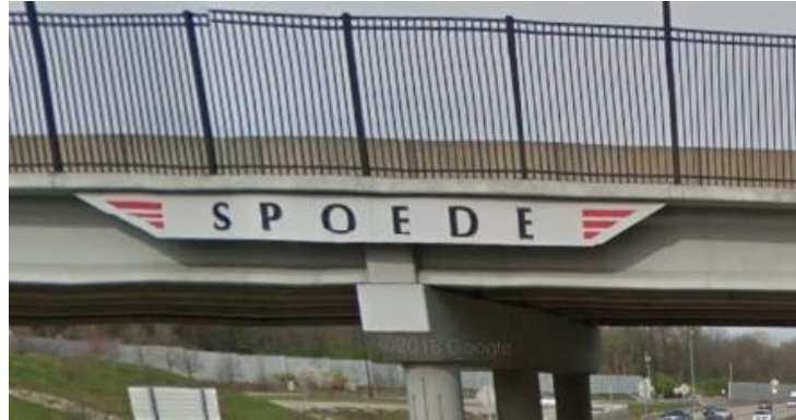
FIG 3.4.1: SIGNAGE ATTACHED UNDER BRIDGE OVERHANG
